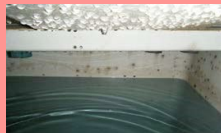
Gel coat (glass reinforced plastic) failure resulting in local biological fouling (dark spots)
