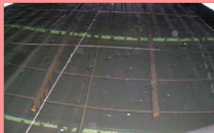
Heavy debris and corrosion of internal parts that will require remedial works
