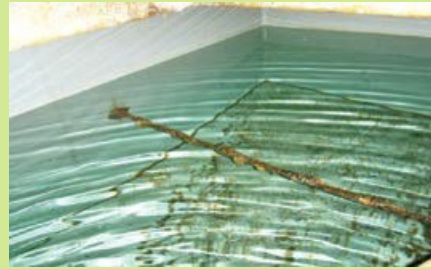
Light debris but corrosion to restraining bars
